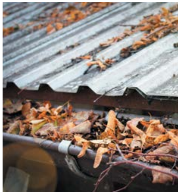
Debris accumulation in gutter.
