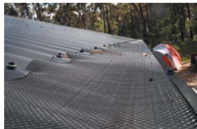
Metallic gutter guard. Source: Paul Whittington
