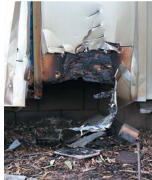
Damaged wall from burning vegetation. Source: CSIRO
