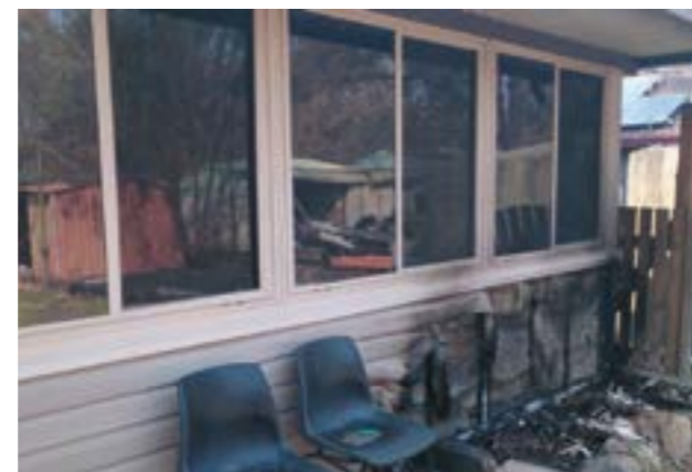
House damage from garden bed burning. Source: CSIRO
