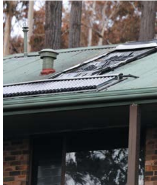
Example of roof perforation and combustible elements on roof.
