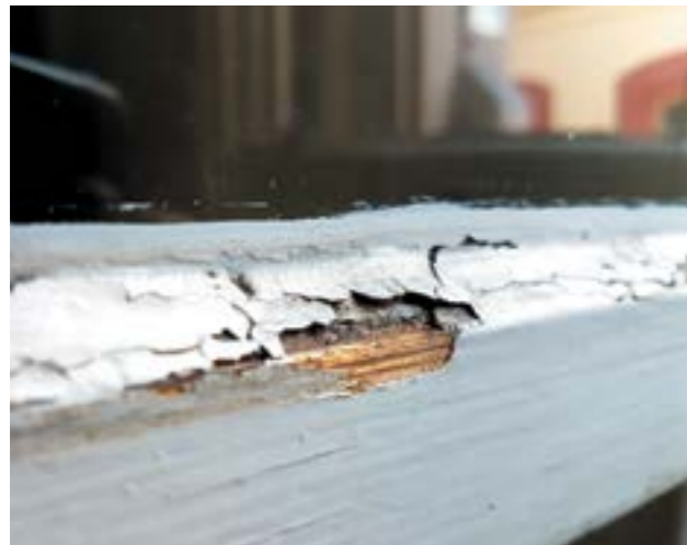
Damaged or decaying timber frames are vulnerable to ember attack.
