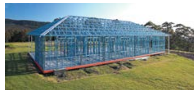
Example of house built using non-combustible framing material (steel frame). Source: KNK Builders
