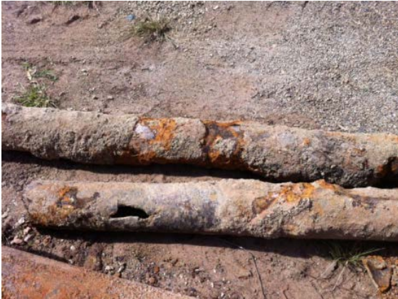
Figure 5 - Typical pipe corroded from exterior
