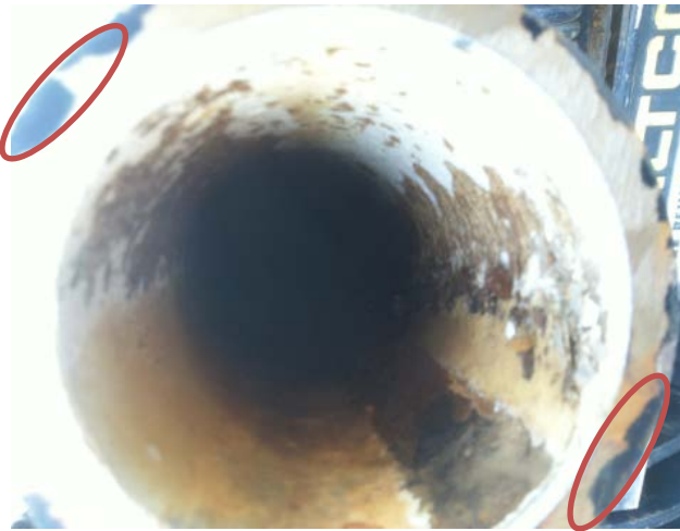
Figure 7 - Pipe showing signs of Carbonisation
