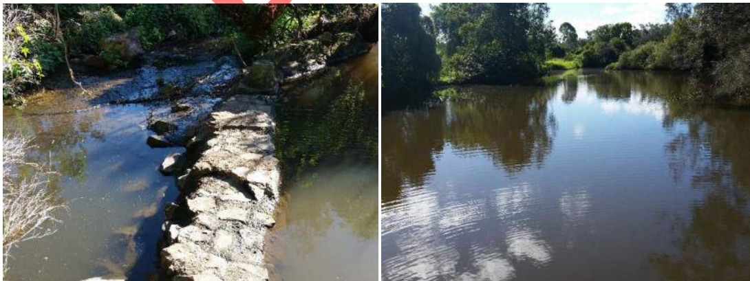
Figure 3-3 Waterbody C – a) Overflow weir, and b) Shallow waterbody upstream from the overflow weir.
