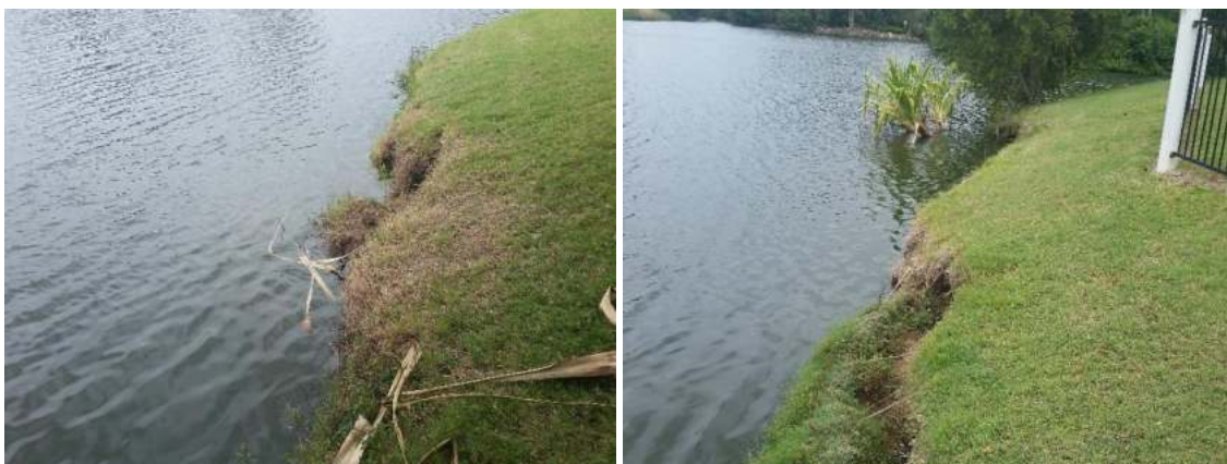
Figure 4-2 Eroded areas within Waterbody C: a) northern edge, and b) near Anembo Drive inlet.
